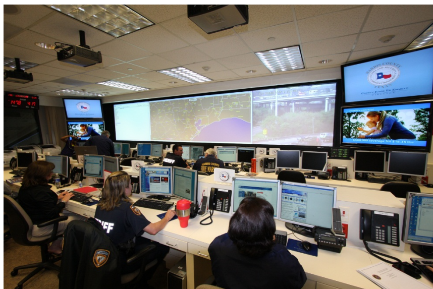
Houston TranStar Emergency Operations Center
